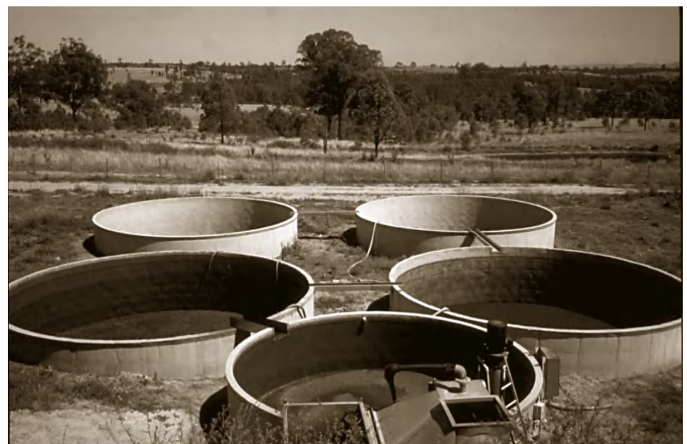
Figure 6. Holding tanks for substrate leachate.
